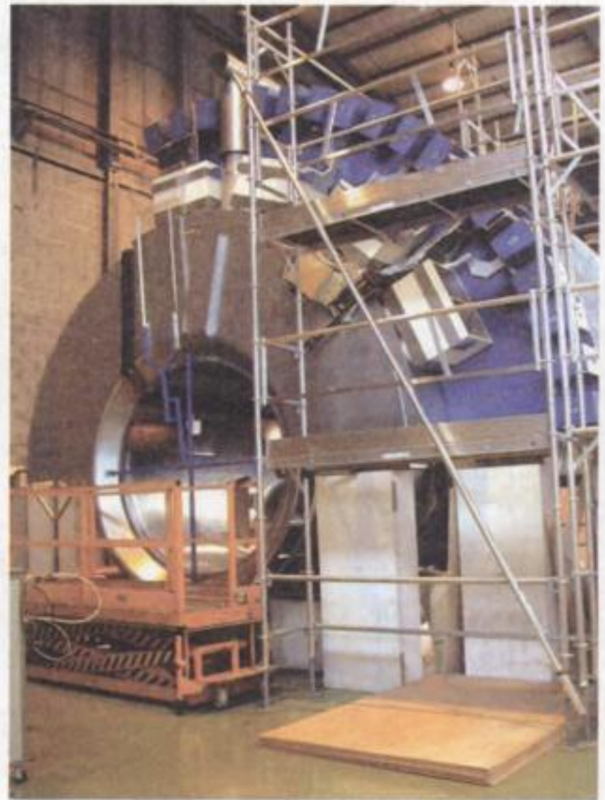
Air evaporative cooling system
